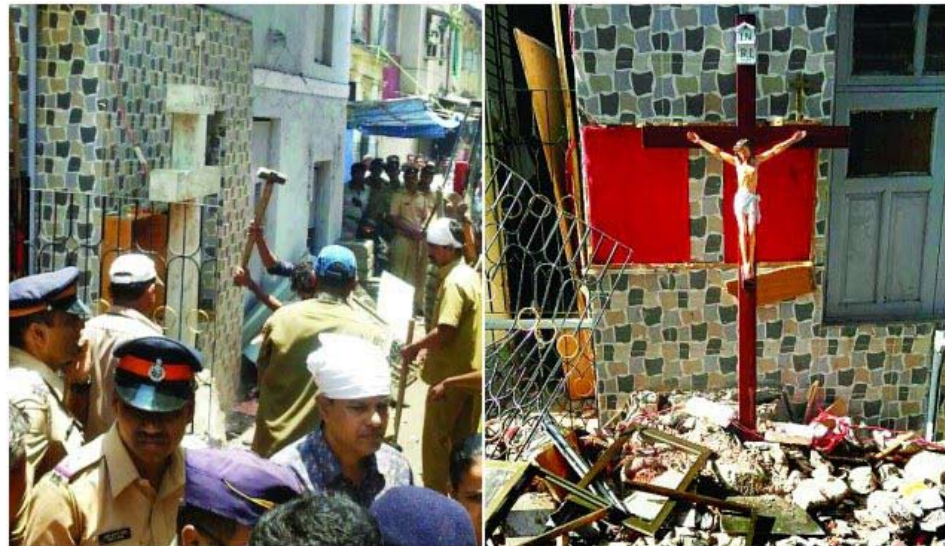
BMC demolishing the Cross; (R) Temporary cross put up at the location by community members
